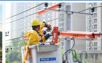
Electric Operation and Maintenance
