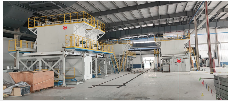
三台化学钢化炉 Three chemical tempering furnaces
